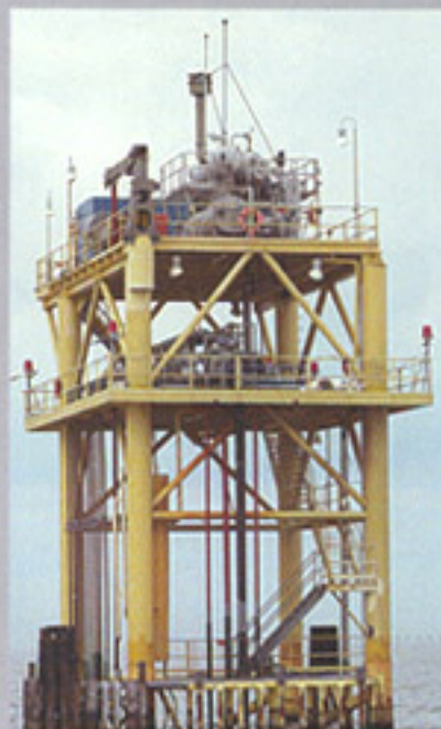
Houston Oil and Mineral, Galveston Bay, Texas. This system has been operating trouble free for fifteen years.
