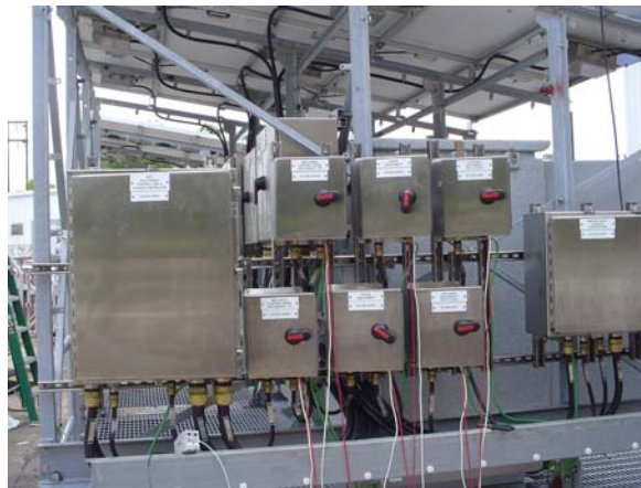
Typical Switch Gear.
