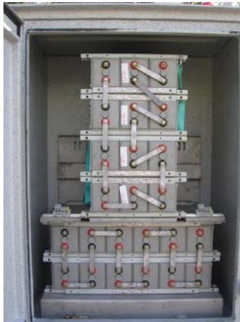
Typical Battery Array.
