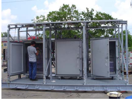
Typical Battery Boxes.
