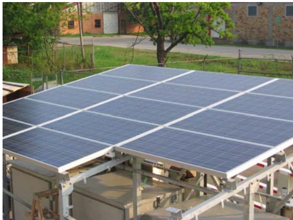
Top View of Array Structure.
