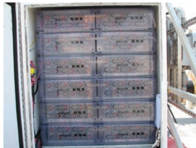
Typical Battery Array
