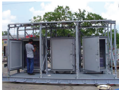
Typical Battery Boxes
