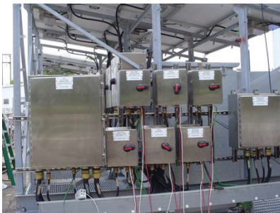
Typical Gear Switch
