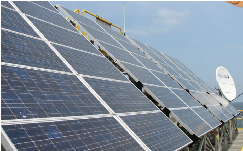
Top View of Array Structure
