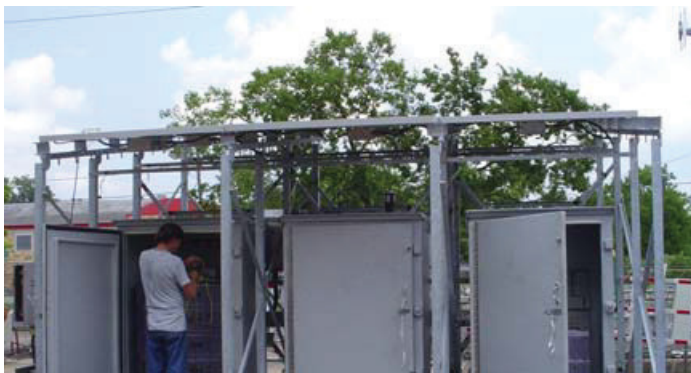
Typical Battery Boxes
