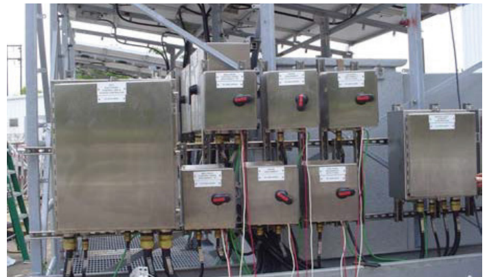
Typical Gear Switch
