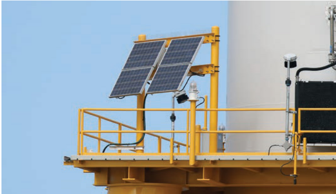
Offshore Wind Farm
