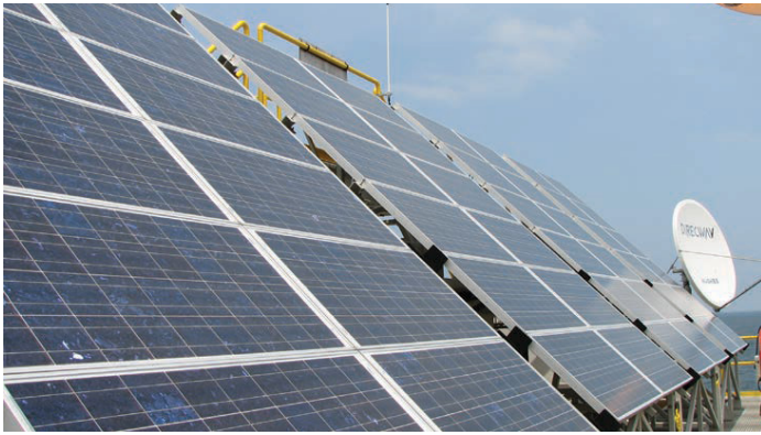
Top View of Array Structure
